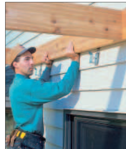
9 Mark the Stratton bracket positions on the ledger to ease alignment, raise the joist assembly and slip the ledger into the brackets for bolting.
