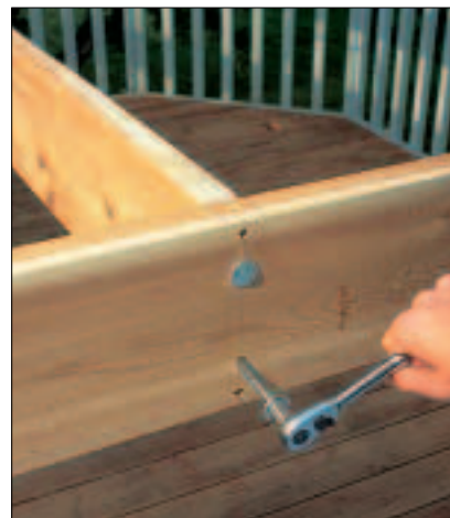
4 Clamp the joists to the ledger with deck screws. Then predrill and reinforce the joints with 3/8 x 5-in. lag screws and washers.
