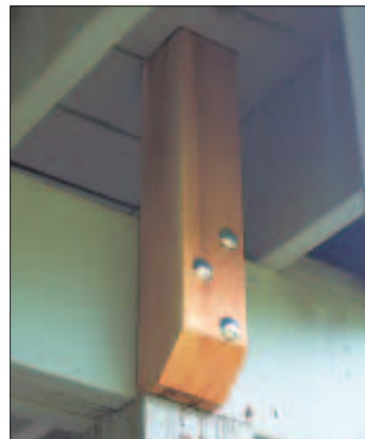
6 Secure each post to the deck's main support beam with three 1/2 x 12-in. carriage bolts; or strap and toenail the posts to the top of the beam.
