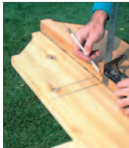
3 After laying out the positions of the joists on the ledger, transfer the marks to the tops of the beams using a combination square.
