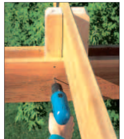
10 After checking the joist assembly for square, secure the free ends by mounting pairs of vertical blocks with deck screws between the beams.
