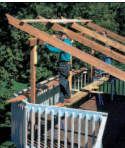
8 Lift the beam and the free ends of the joists simultaneously and rest the beam on support blocks for bolting. Note the temporary bracing.
