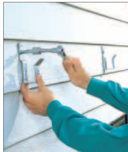
5 Predrill and bolt the Stratton brackets to the house to support the ledger board. Position the brackets so you drill into solid house framing.
