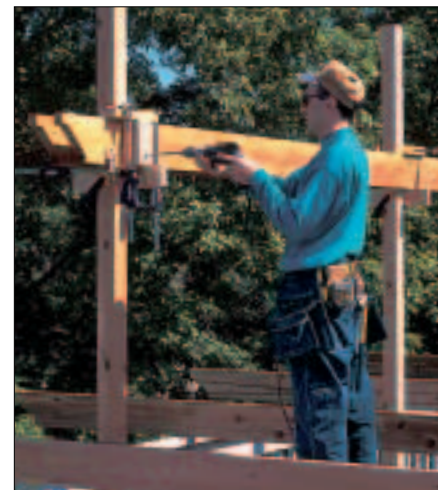
7 Temporarily clamp the pergola's saddle beam to the post and predrill for bolts. A simple wooden alignment jig ensures uniform and straight holes.
